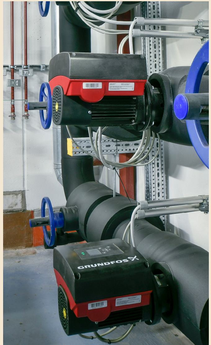
Cold water pumps for pumping the cold medium to the Zortström distributor
