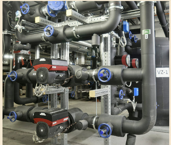
New cold power supply center with one of three Zortström distributors and cold pumps
