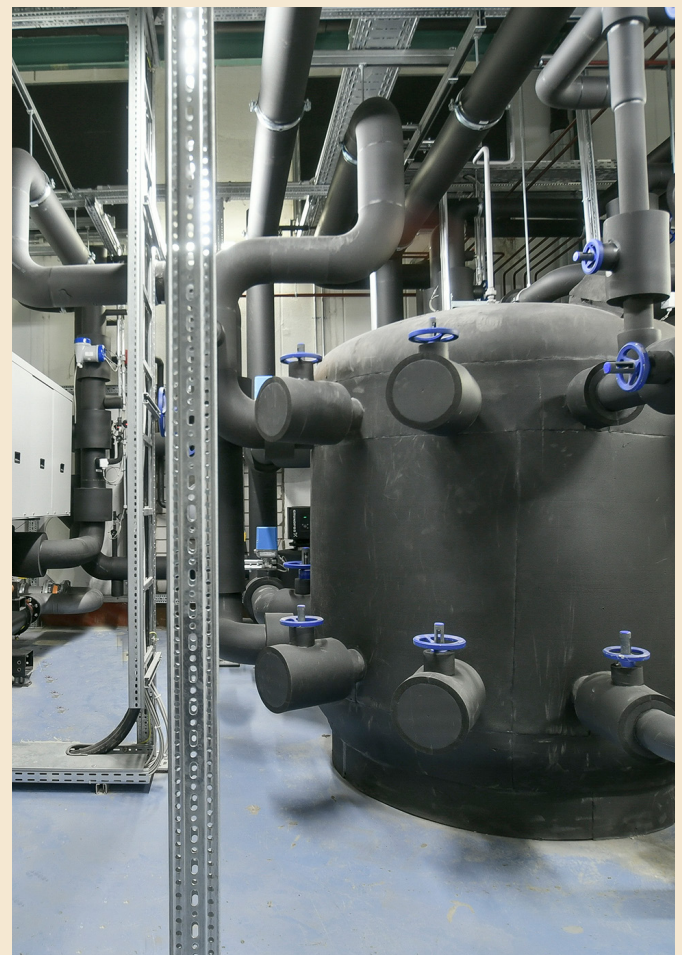
Refrigeration unit and one of the three Zortström distributors installed
