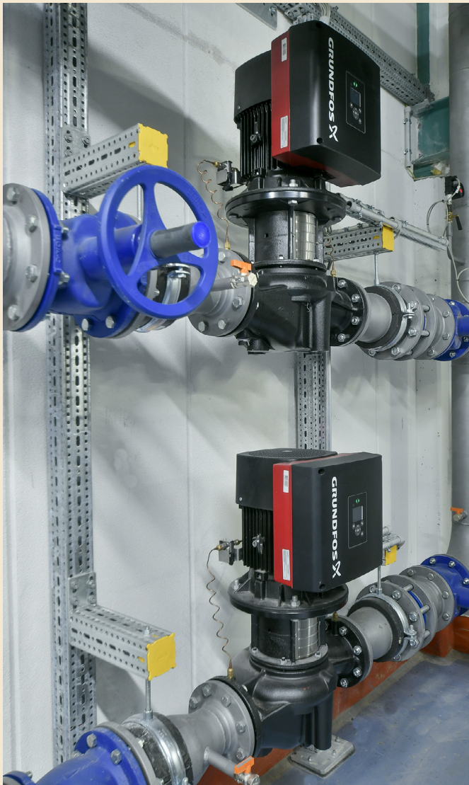
Pump system for pumping the cooling water to the dry cooling tower
