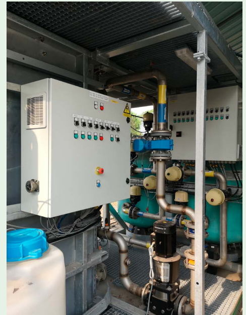
The main plant
