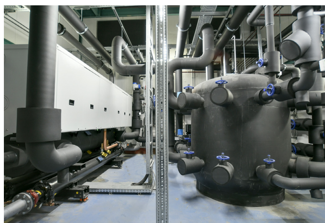
Refrigeration unit and one of the three Zortström distributors installed
