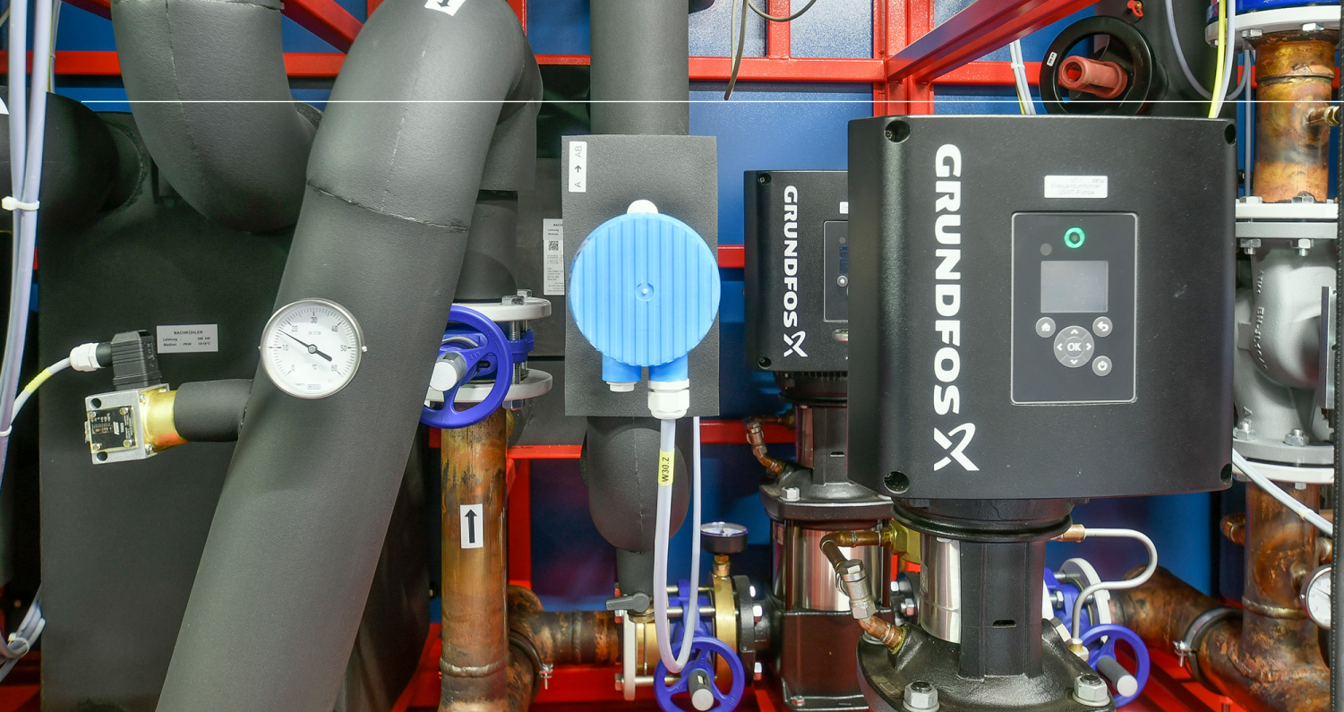
Group of fittings from the high-efficiency SEW heat recovery system
