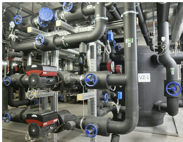
New cold power supply centre with one of three Zortström distributors and cold pumps
