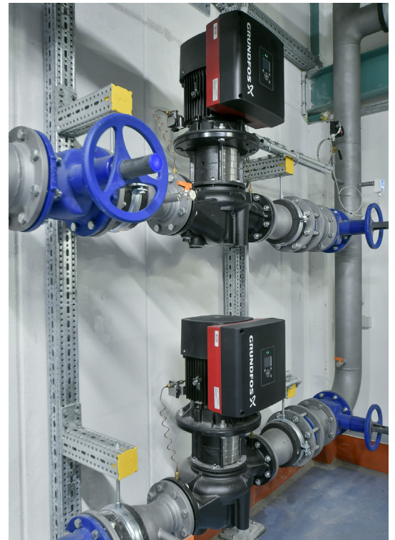
Pump system for pumping the cooling water to the dry cooling tower
