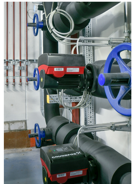
Cold water pumps for pumping the cold medium to the Zortström distributor
