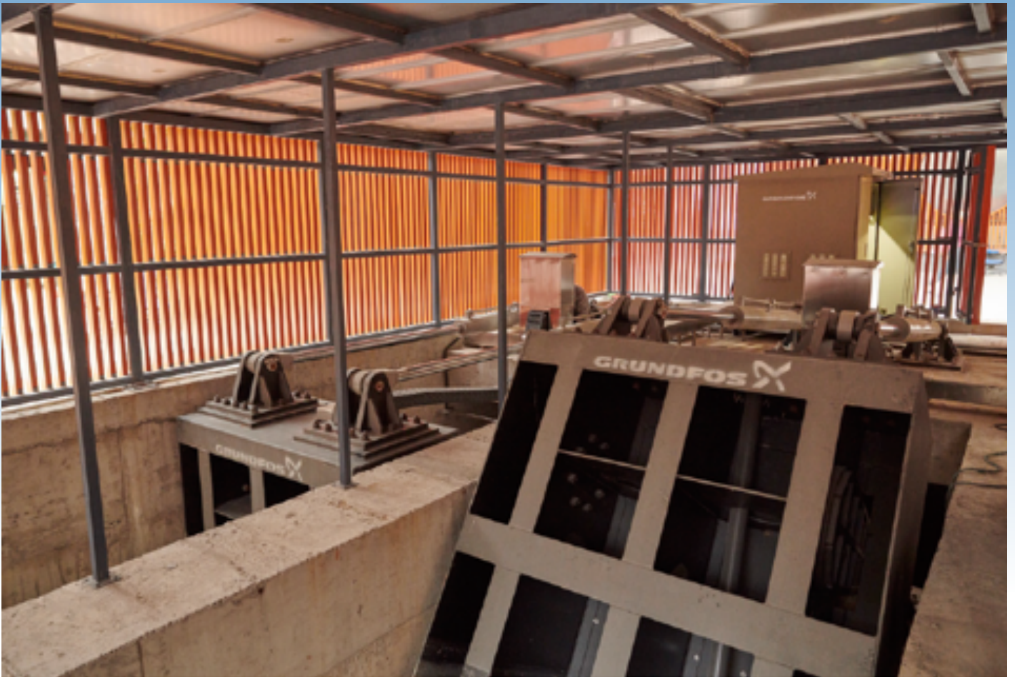
Grundfos pump gates in Fuzhou, China
