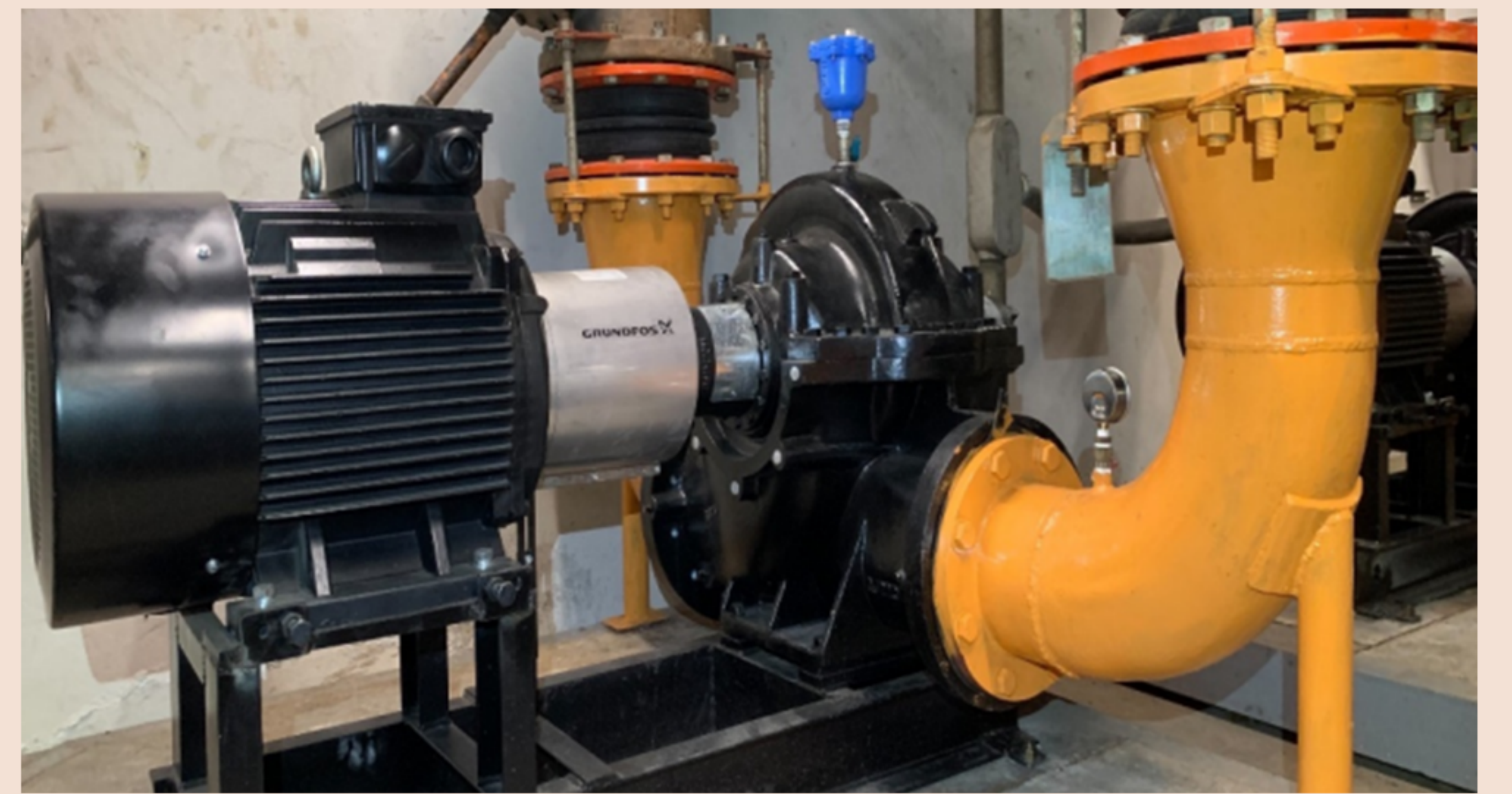
Grundfos Chiller Condenser Water Pump
