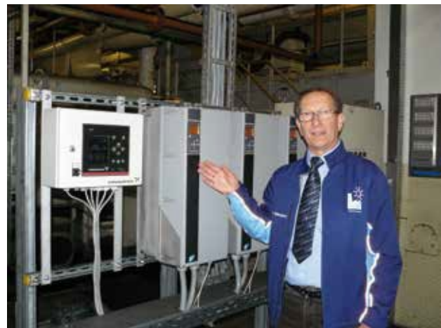
"Only the newly installed control technology is capable of recognizing when the machine tools need less or no cooling lubricant and therefore the pumps can be stopped completely" (Paul-Gerhard Römermann, Energy Officer at Volkswagen AG's Braunschweig plant).
